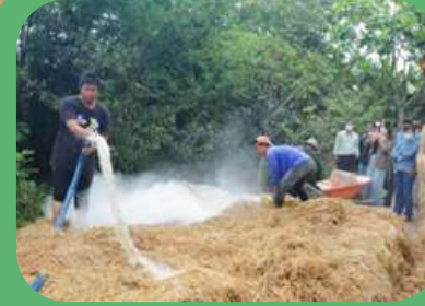
Spread a thin layer of burned lime alternating with a layer of straw
